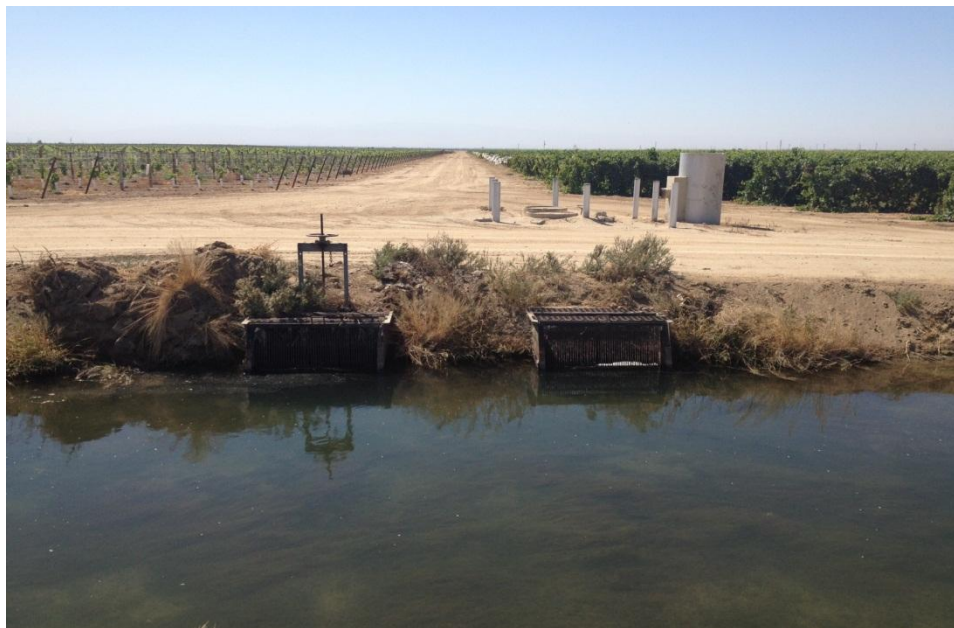
Figure 10. Typical North Kern Irrigation Turnout.
